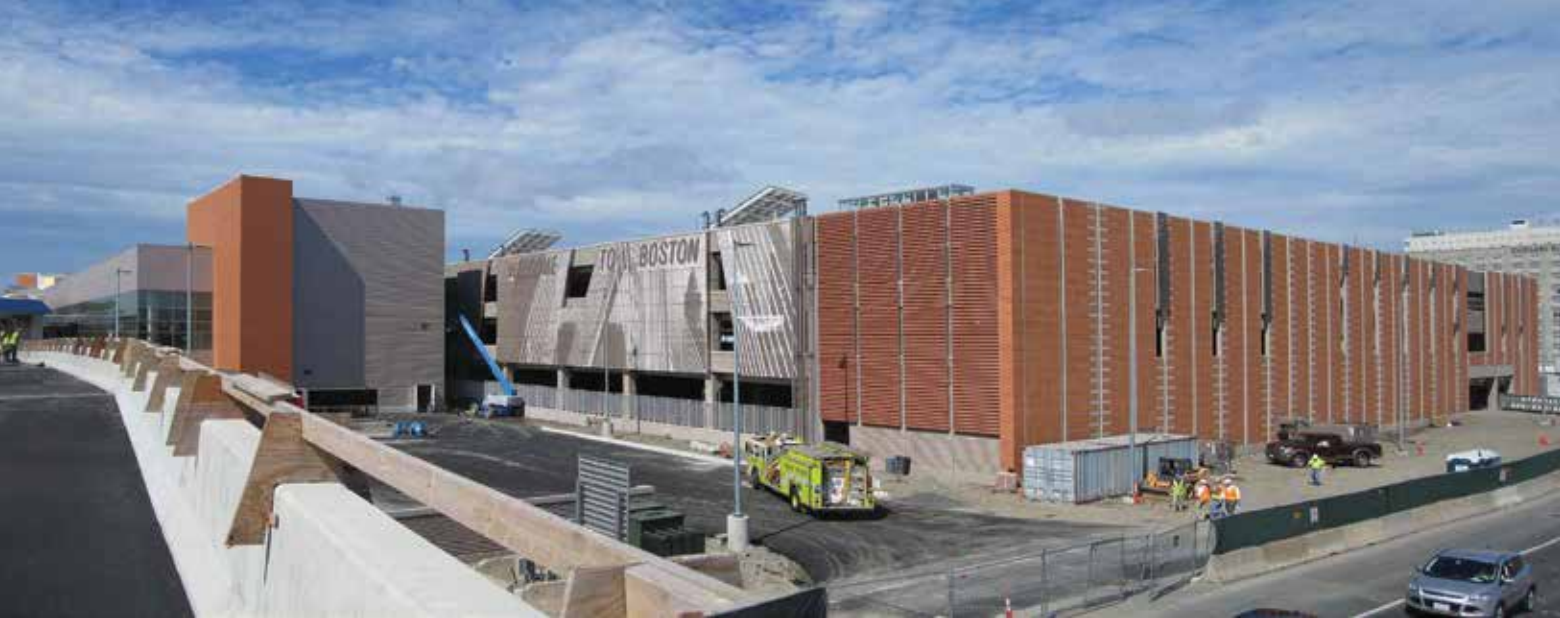
Precast concrete components created 60- by 60-foot bays for the CONRAC facility at Logan International Airport in Boston, Mass. Structural H-frames supported loads along the perimeter, with interior moment frames used between columns and tees. Terra cotta veneer was applied to the exterior, its first use in North America on structural components. Photo: Fennick McCredie Architecture.
